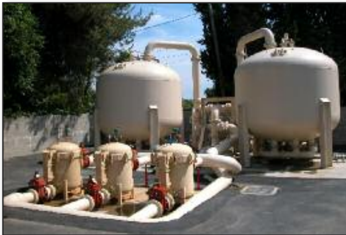
Lincoln Ave. Water Co. treatment facility
