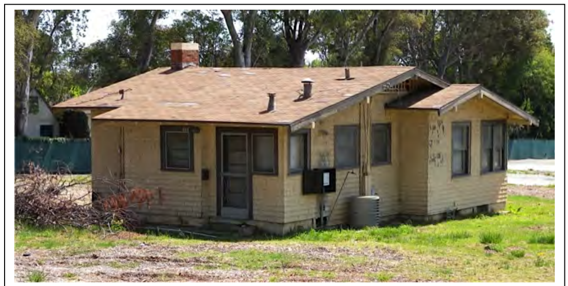
Below: The only building left on the property, "Gloria Cottage" awaits its fate.
